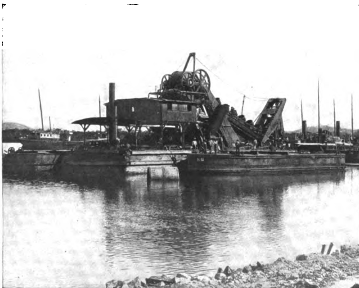
ONE OF THE GIGANTIC DREDGES AT WORK AT THE TERMINUS OF THE PANAMA CANAL
