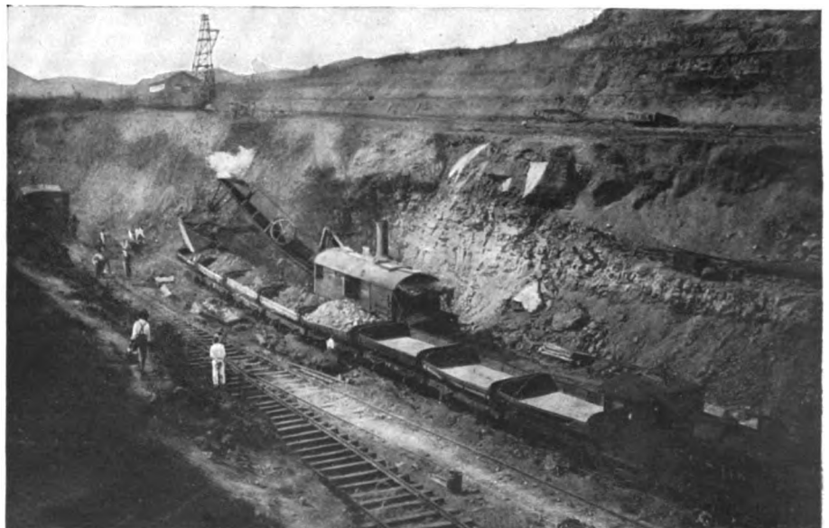
THE GREAT CULEBRA CUT ON THE PANAMA CANAL. HERE IS SHOWN ONE OF THE GIGANTIC STEAM SHOVELS AT WORK FILLING CARS
