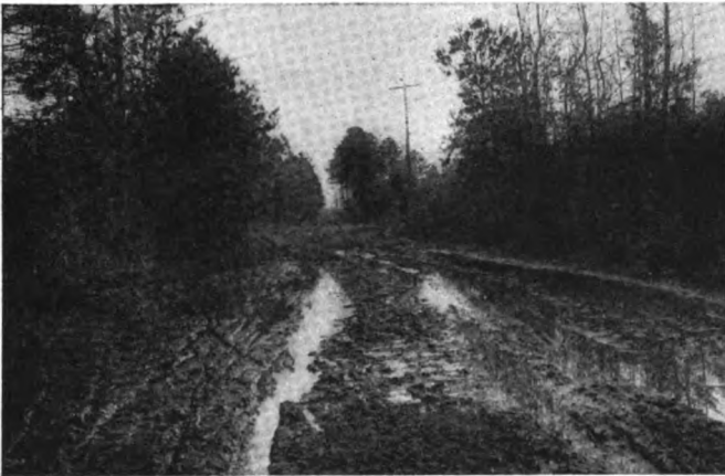
A ROAD IMPROPERLY CONSTRUCTED
