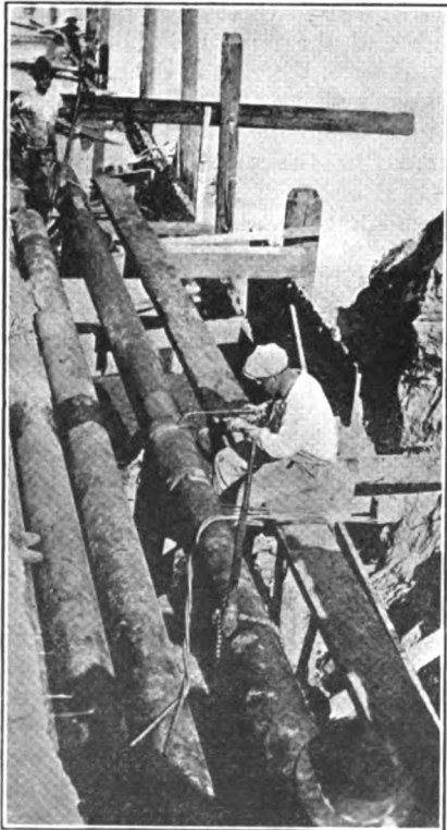
FIG. 2.—HOW THE PIPE WAS WELDED INTO 100-FOOT SECTIONS ON THE BANK OF THE RIVER
