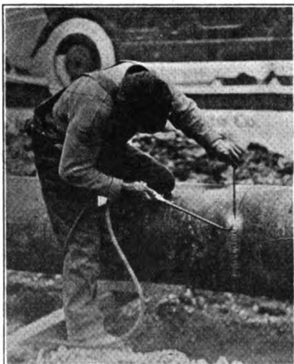
WELDING GAS LINE JOINTS SHOWS BIG ECONOMY. THIS SHOWS A 14-INCH LINE BEING WELDED
