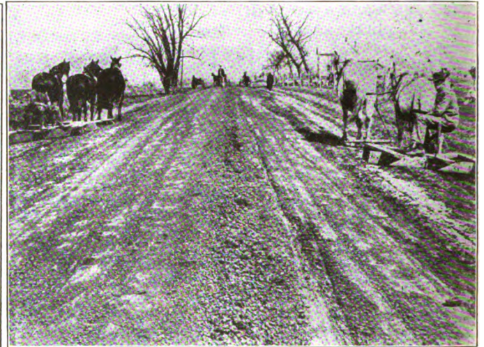
WHEN THE SPLIT-LOG DRAG IS USED AS IT IS BEING USED ON THIS ROAD, THE SURFACE BECOMES RUTLESS AND HARD. NOTE THE STONE DRAGGED TO THE CENTER
