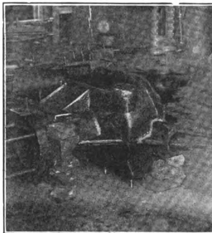
Fig. 1. SHOWING THE LOCATION AND EXTENT OF THE FRACTURE "V" GROOVING AND MANNER OF HOLDING BROKEN PARTS IN PLACE
