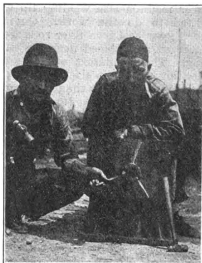
FIG. 1.—THE METAL WAS CUT AWAY FROM BOTH SIDES OF THE CRACKS IN A V-SHAPED GROOVE.
