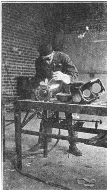
FIG. 1.—THE BROKEN FLANGE WAS WELDED FIRST AND WITHOUT PREHEATING.
