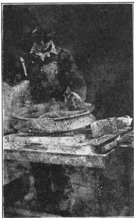
FIG. 2 THE FIRECLAY BACKING USED TO SUPPORT THE BROKEN FLANGE WHILE SPOT WELDING IT
