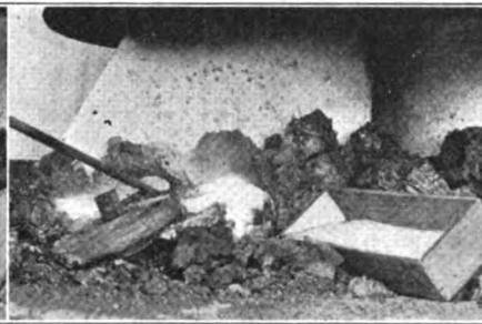
FIG. 10—AND THEN THE SPELTER IS PUT ON TO RUN INTO THE JOINTS
