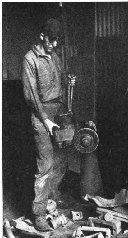
FIG. 1.—THE CRACK WAS GROOVED OUT AND THE SURFACE CLEANED WITH THE WIRE BRUSH
